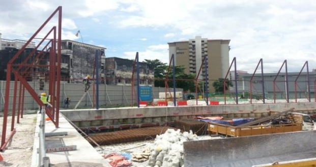
▲ Malaysia KVMRT – Cochrane Station
